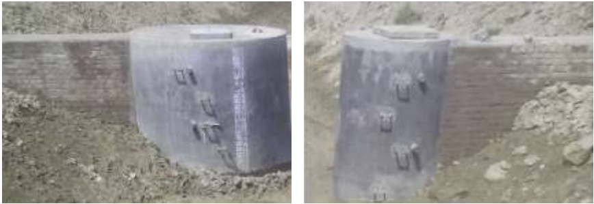
Fig. 7. Modified Recharge wells for measurement of water recharge rate
