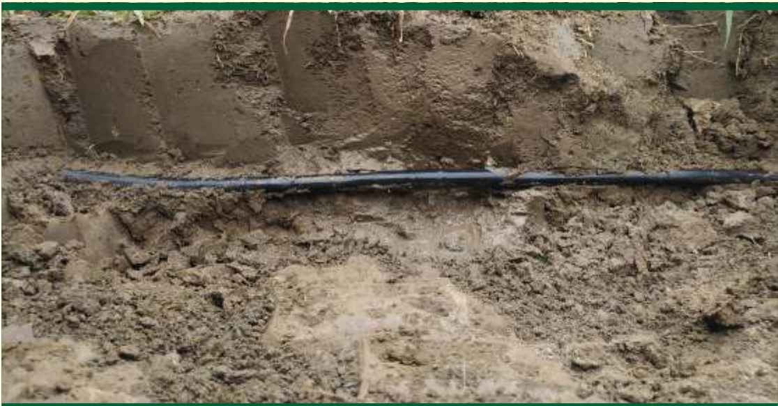
Plate-4 Drip line view under subsurface of soil
