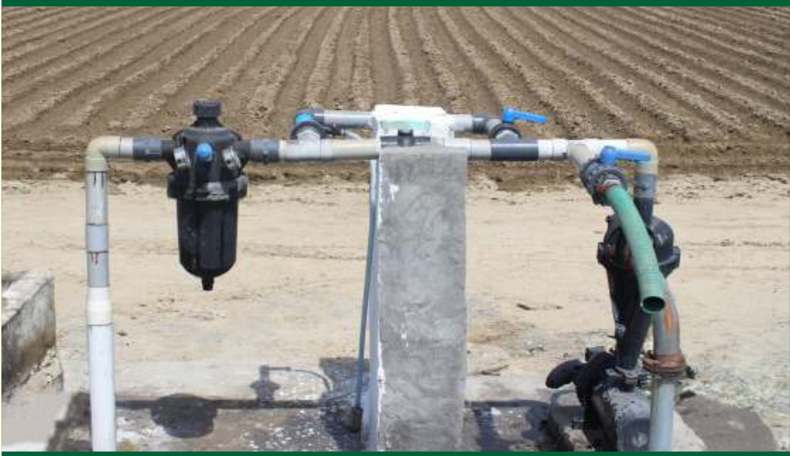
Plate-3 Pumping unit
