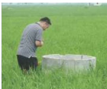
Installation of SSD system and bumper paddy crop during post SSD project at village Jagsi (Sonipat)
