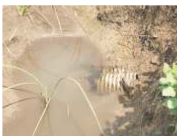
Poor condition of drain pipes and open surface drains
