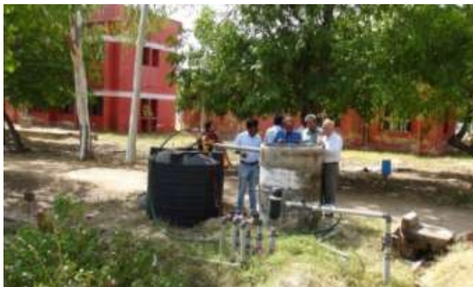
Plate 2: Gypsum bed treatment for alkali water
